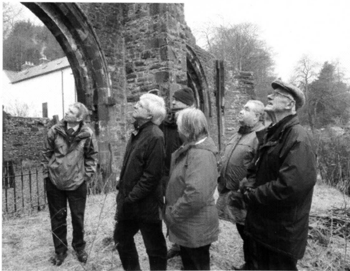
March 2015: Trustees inspecting problem areas in the abbey church walls
